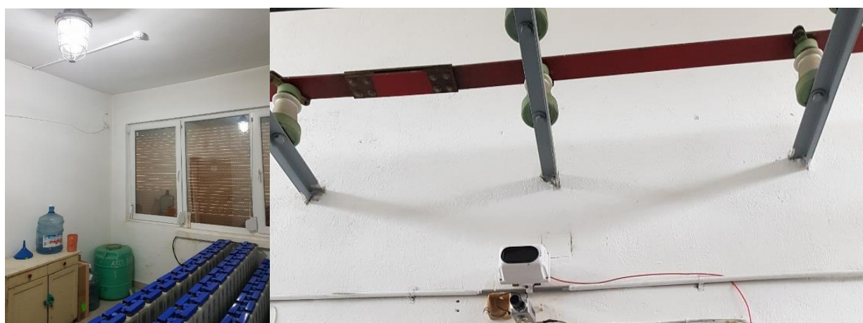
Figure 3: Fire detection in batteries room and middle voltage part
