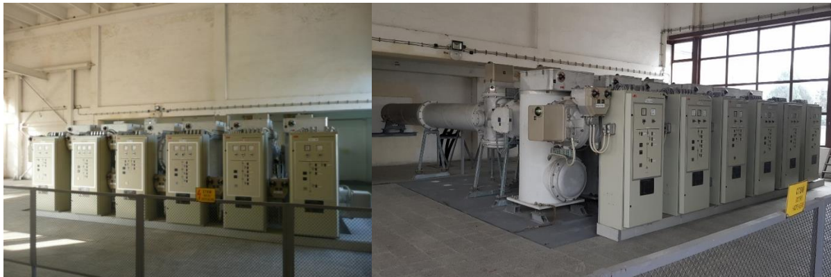
Figure 4: 110 kV enclosed part
