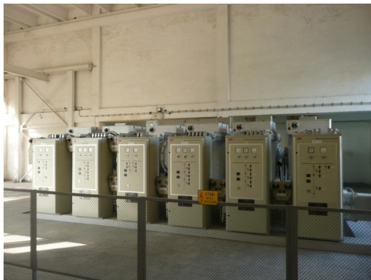
Picture 9: 110 kV enclosed part
