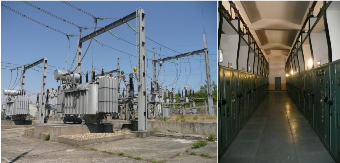
Picture 4: 110 kV and 10 kV part
