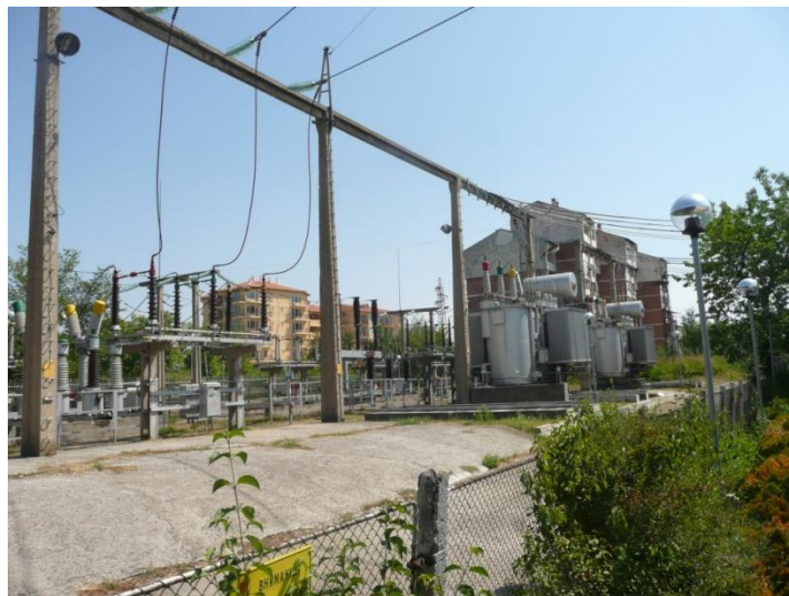
Picture 7: Veliko Tarnovo substation
