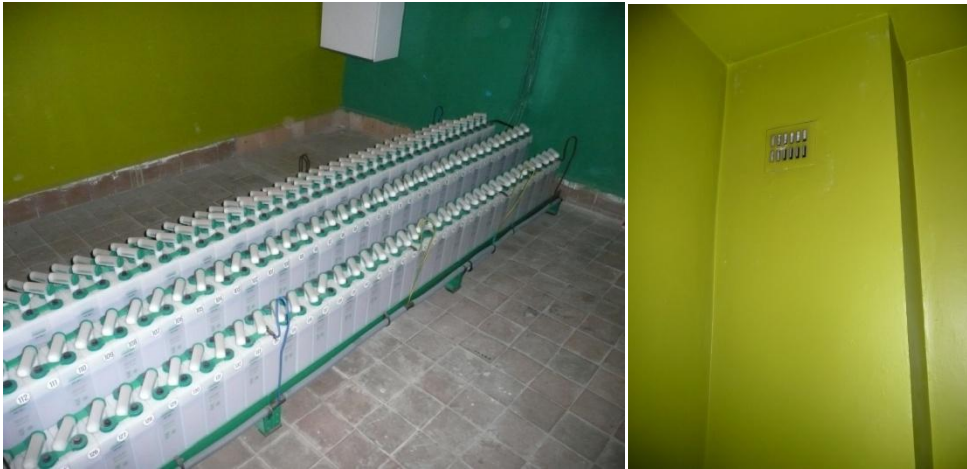
Picture 6: Backup bateries
