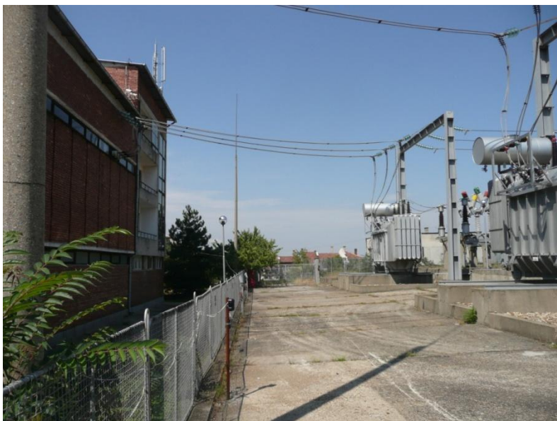
Picture 5: Kartala substation
