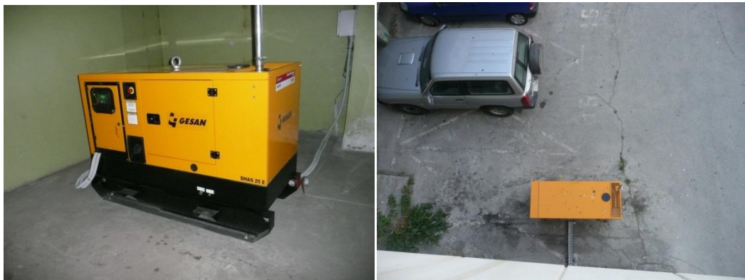
Picture 10: Diesel generators in Gorna Oriachovitsa and Varna
