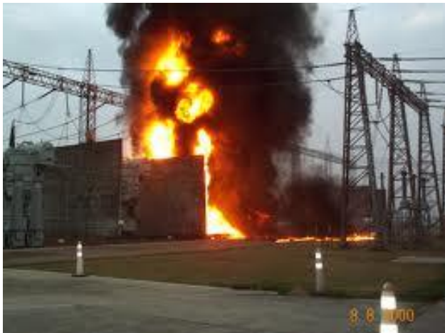
Picture 1: Illustration picture how can transformer burn
