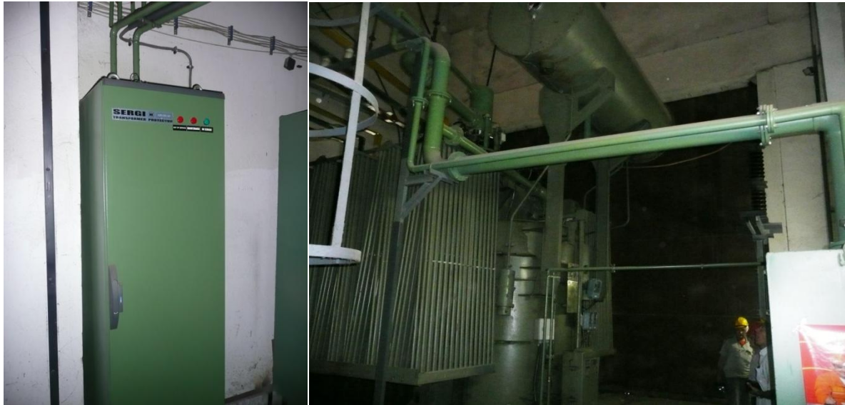
Picture 13: Sergi extinguishing system
