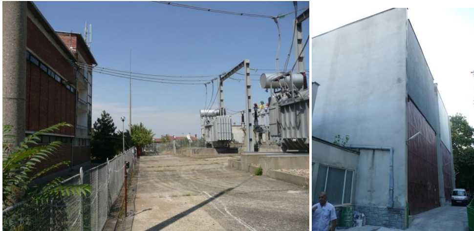
Picture 2: Kartala and Čajka substation
